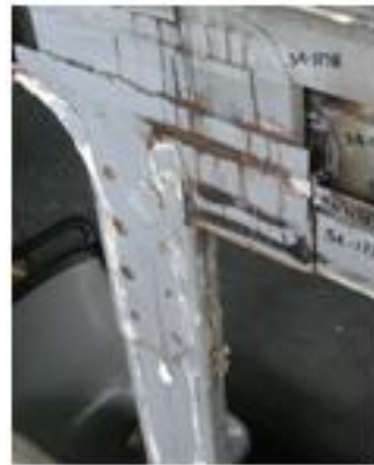
Figure 4: Failure of the bus structure
