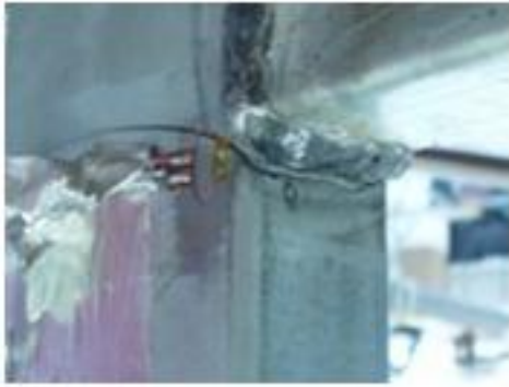
Figure 9: Crack resulting from the fatigue testing, right side of the specimen test
