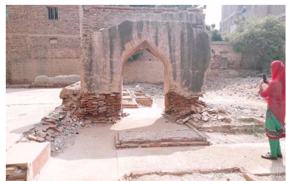
Figure 2: Deteriorated condition of Mir's Tomb site, Source: Author
