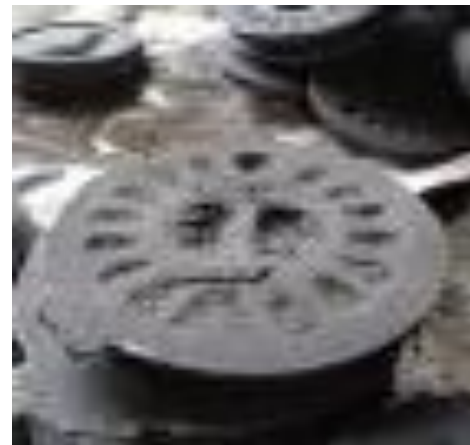
Figure 4: Example of Deformation Defect
