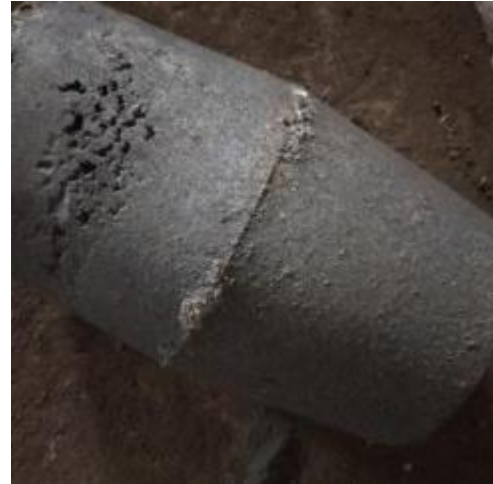
Figure 3: Example of Cohesive Defect
