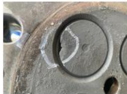
Figure 2: Valve damage (perforated and broken)
