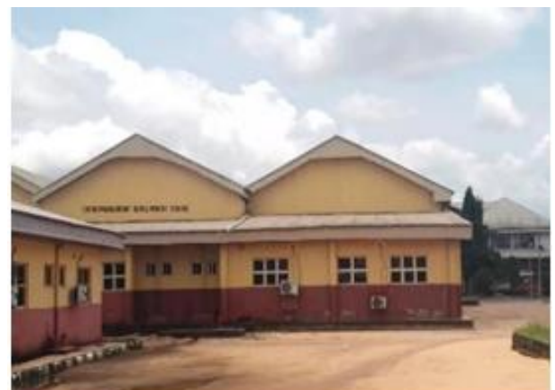
Plate 4 – Effect of rising damp on walls
