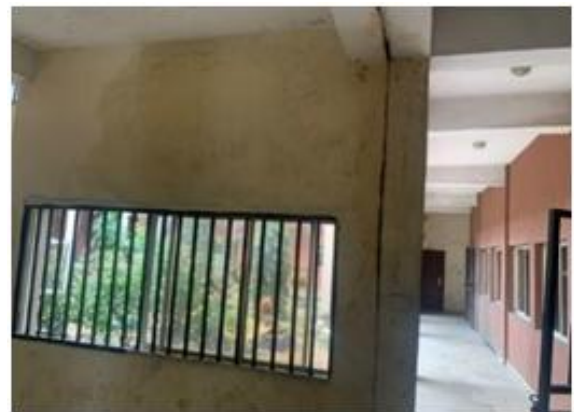
Plate 2 – Moisture through expansion joint
