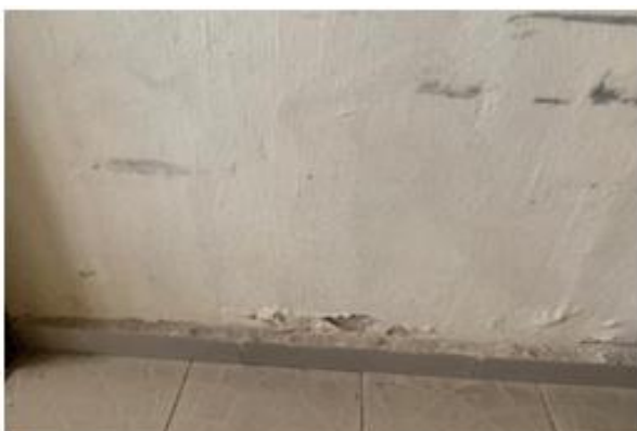
Plate 1 - Flaking of paint on interior wall
