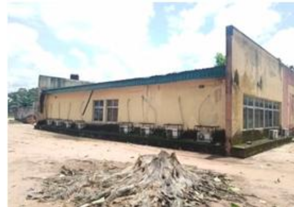
Plate 3 – Moisture action on unprotected wall
