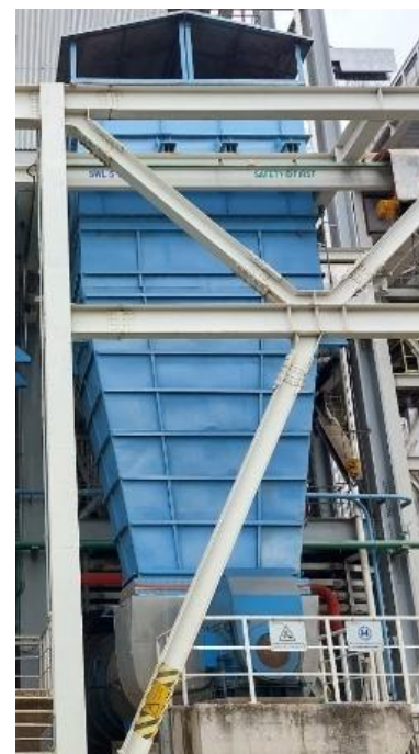
Figure 1: Forced Draft Fan in a Power Plant
