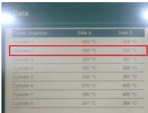
Figure 2.2: Temperature reading on the Gas Engine Chamber by the PLC
