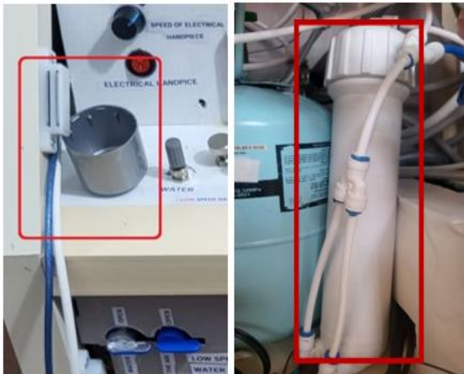
Figure 3: Illustrates the water tank on right side, while on the left side designated filling location, and valve configuration under the cup
