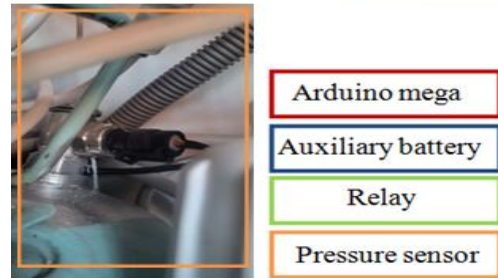
Figure 4: The Elements Comprising the Control Circuit, Encompassing the Arduino, Relay, and Pressure Sensor
